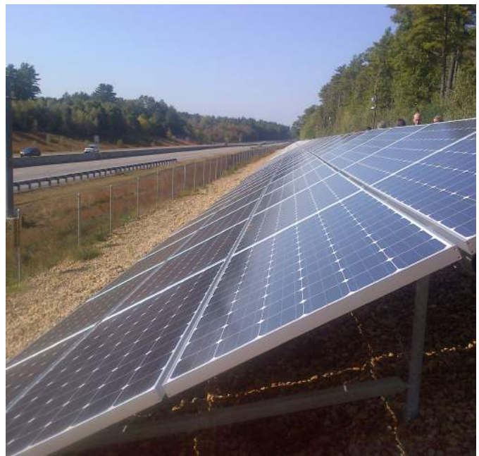
Solar energy has grown rapidly in Massachusetts in recent years. Pictured here is a solar installation along Route 44 in Carver, Mass.
